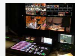
Live Production System at New World Symphony
